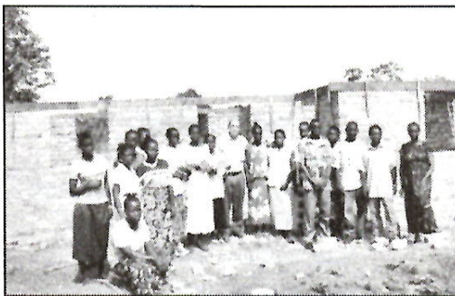
The women proudly gather. The trusses and roof will be next on the Resource Center.
